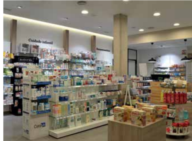
Compatible lighting with installations that require UGR<19
