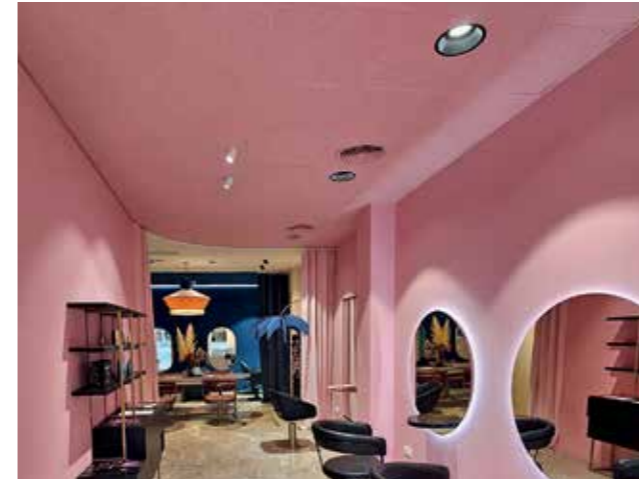
Compatible lighting with installations that require UGR<19
